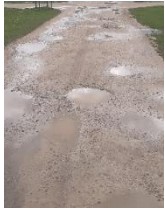
Image 4. An example of path erosion
