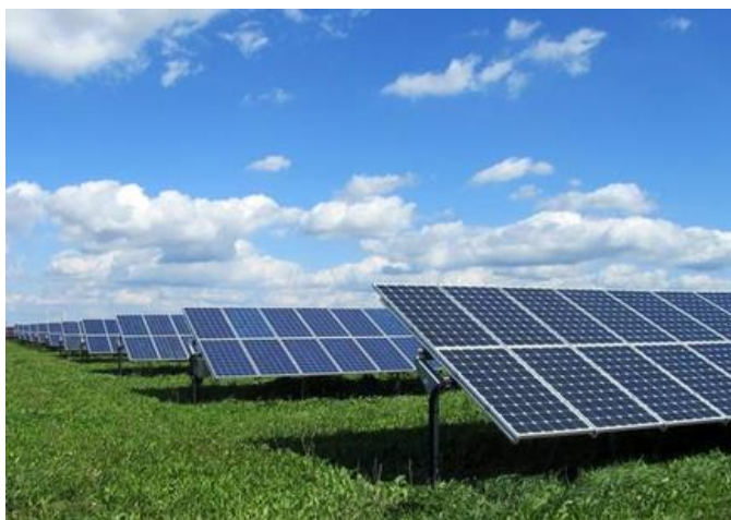
Commercial Ground Mounted Photovoltaic
