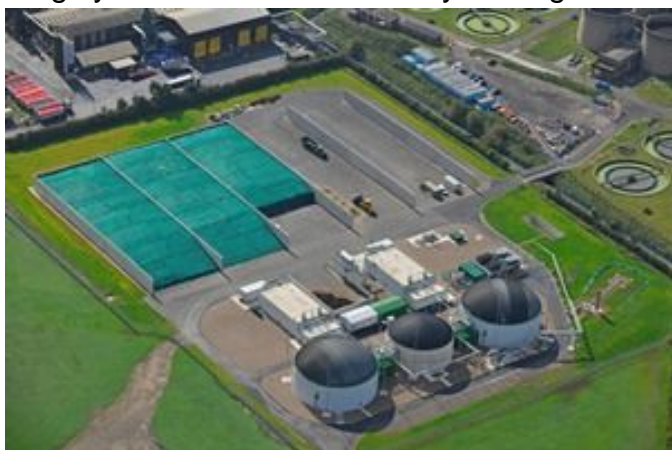
Figure 4: Stoke Bardolph Anaerobic Digestion Plant http://www.edie.net/news/4/Severn-Trent-Water-to-invest-in--15m-AD-plant/
